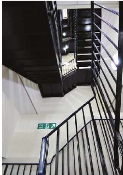
A stairwell at Cavendish Mill, an apartment block owned by New Charter, before and after LED luminaires were used as part of trials to test the technology.
